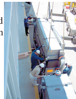
Exciting things are happening: Workers deliver a new chiller system at Harbor College.
